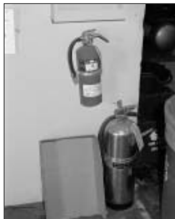
Know where fire extinguishers are located and how to use them.
