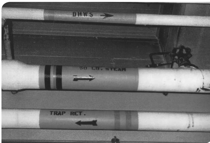
Hazardous products in pipes identified by colours and letters
