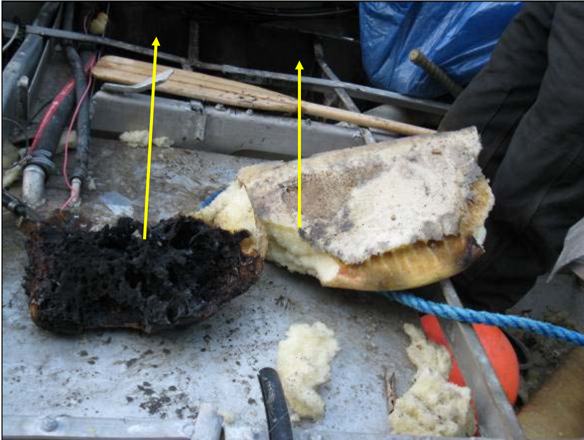
Figure 9: Flotation foam removed from the hull of the boat. The arrows point to where the investigator removed the pieces of foam. The bottom surface of the charred foam was more burned where it had contacted the surface of the hull.
