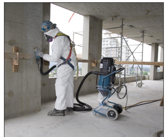
Worker grinding concrete using a HEPA vacuum exhaust attachment on the grinder.
