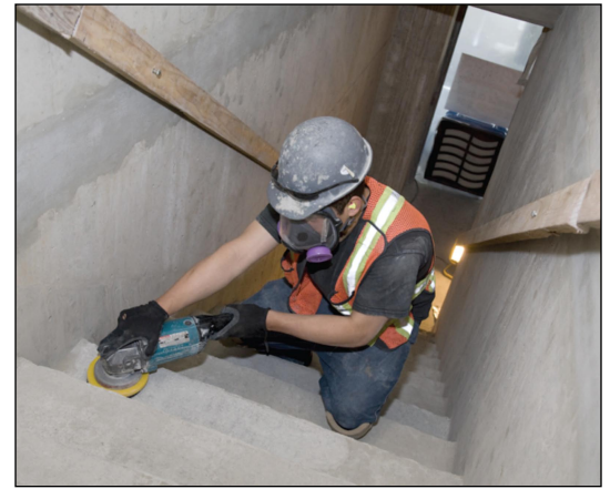
Worker grinding concrete in a stairwell with local exhaust ventilation. Note the exhaust unit at the bottom of the stairs.
