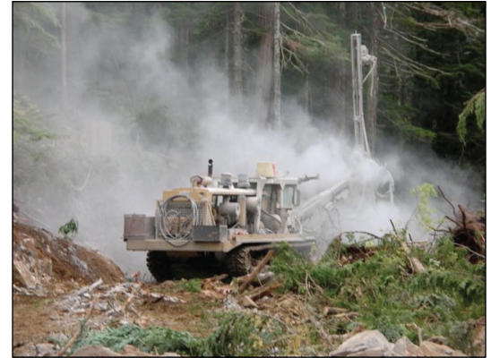
Rock drilling without dust controls.
