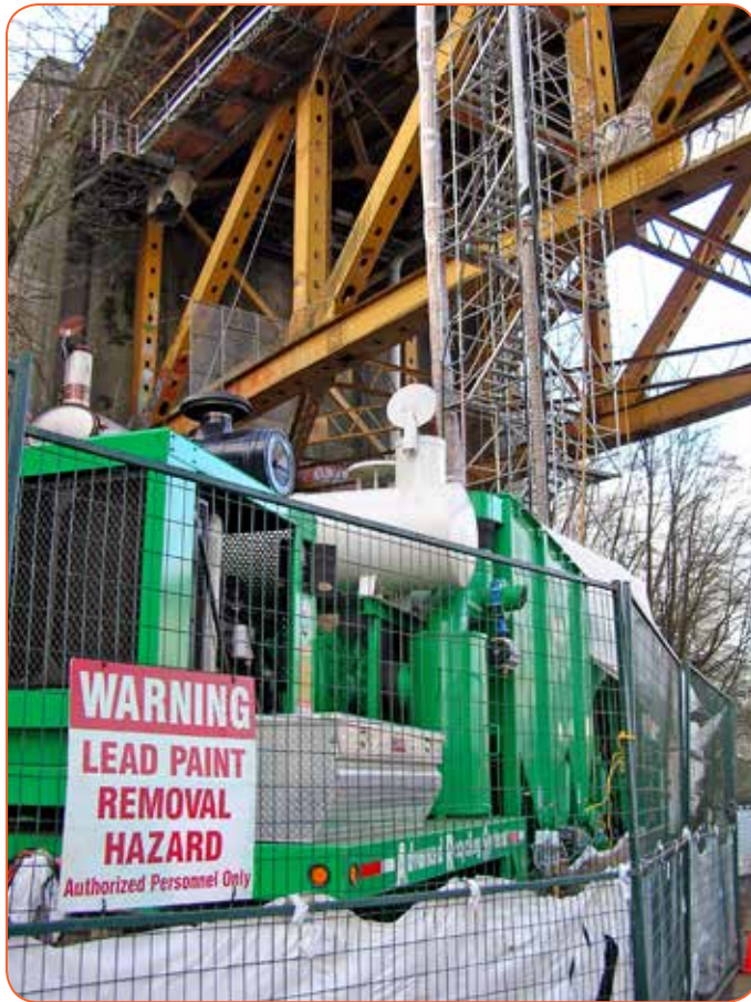
Fence and warning sign on a lead removal site
