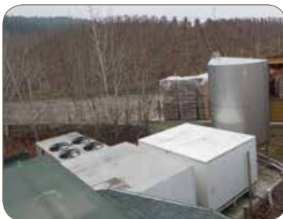
Clean-water storage tanks
