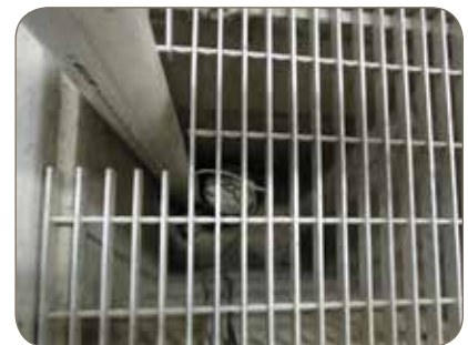
Sump with pump
