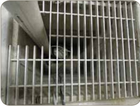
Sump with pump
