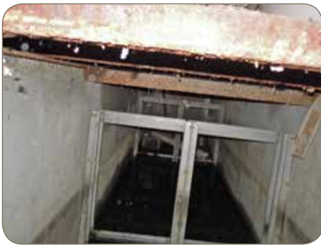
Black-water storage tank
