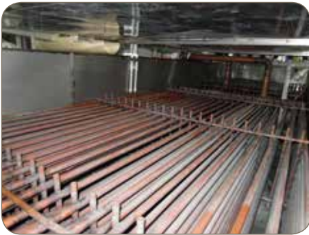
Heat exchanger tank
