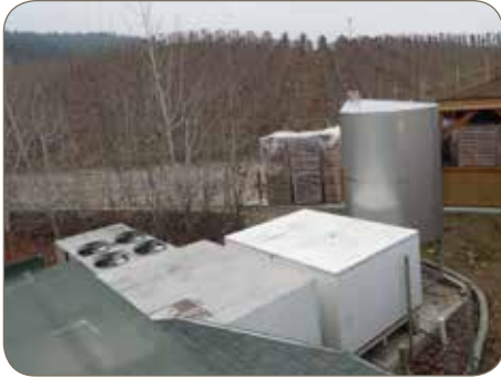
Wash-water storage tanks (square) and rainwater storage tank (round)
