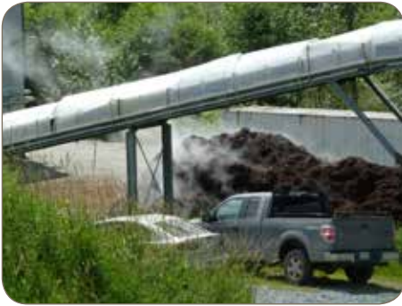
Covered conveyor system
