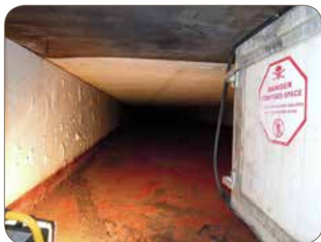
Pasteurization tunnel (crawl space)
