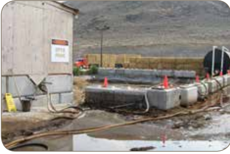
Pump shed and composting pond
