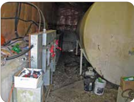
Water tank inside a shed
