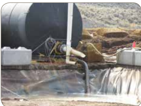
Brown-water tank feeding a compost pond
