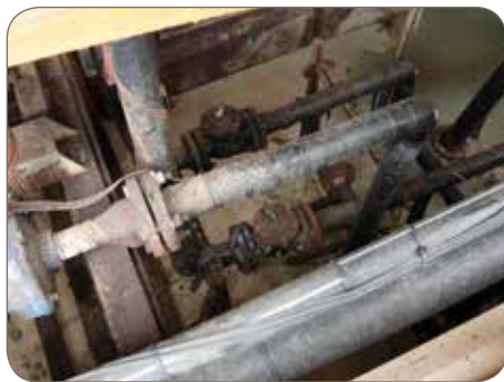
Piping inside a pump shed
