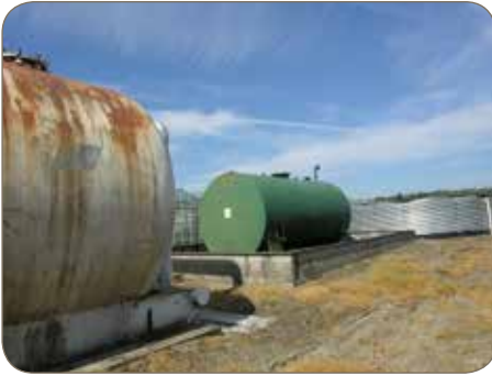
Above-ground steel fuel tanks
