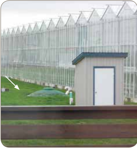
Septic tank hatchways
