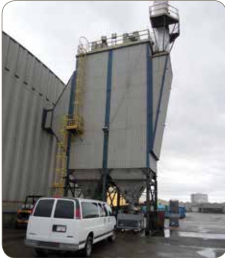
Wood-fired boiler system
