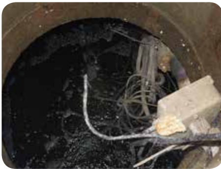
Pump station in a greenhouse
