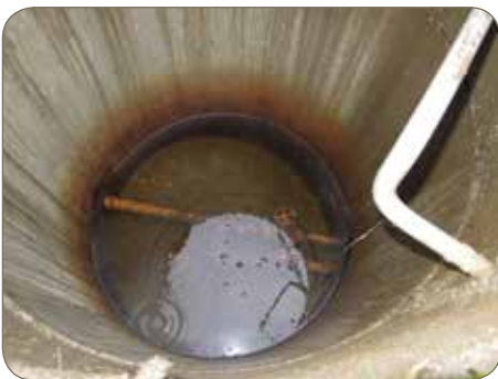
Below-ground valve chamber
