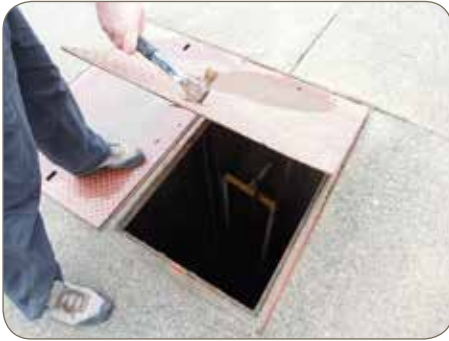
Lift station hatchway
