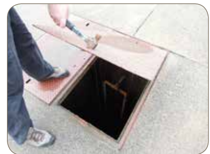
Lift station hatchway
