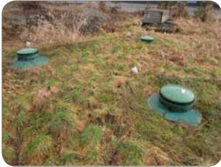
Septic tank hatchways
