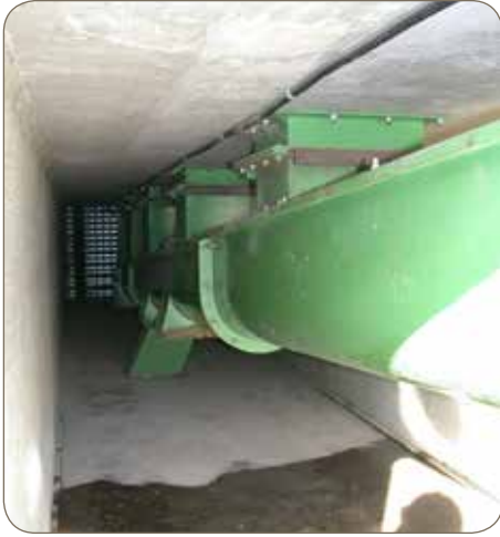
Conveyor in a tunnel
