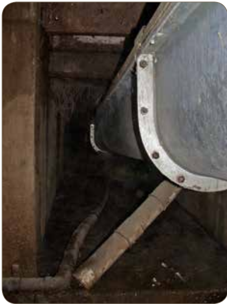
Conveyor in a tunnel
