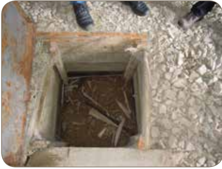
Below-ground valve box
