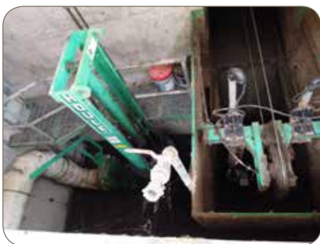
Liquid-manure pump chamber
