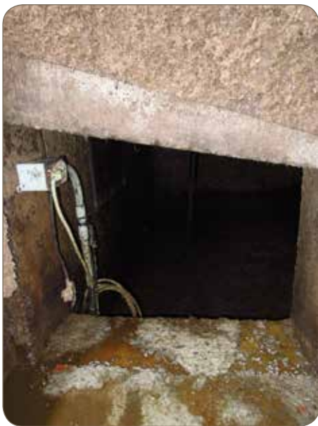
Liquid-manure pump station
