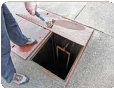
Lift station hatchway
