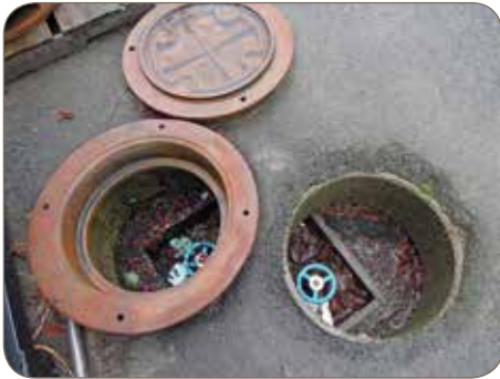
Stormwater manhole and drains
