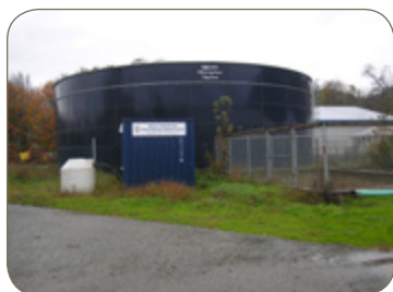
地面上蓄糞槽
