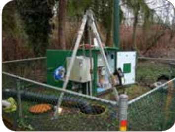
Entry and ventilation equipment setup
