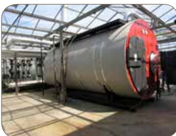
Boiler in a greenhouse
