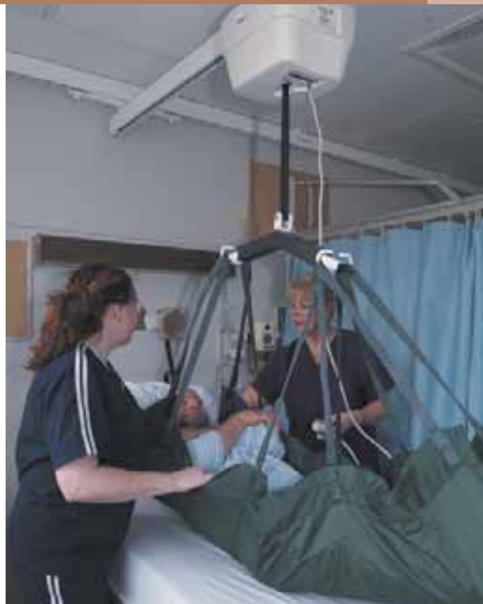
Registered nurse Patti Peach (left) and licenced practical nurse Sharon Mathieson (right) demonstrate the ceiling-mounted lift system that has reduced MSIs in the Neurosciences Unit at Lions Gate Hospital.
