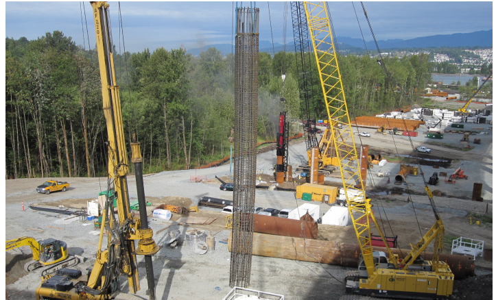
Surrey - The new bridge abutment construction area, adjacent to the existing Port Mann Bridge.
